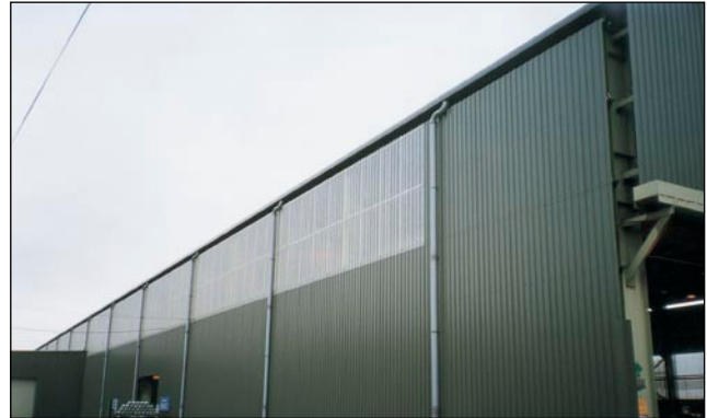
Figure 43 Lighting panels installed in the wall rather than the roof
