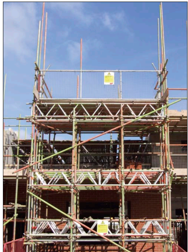
Figure 35 Loading bays should be designed for the actual weight of the materials to be placed on them and include an additional allowance for impact loads from mechanical handling (eg cranes or forklifts). A notice should clearly display the safe working load
