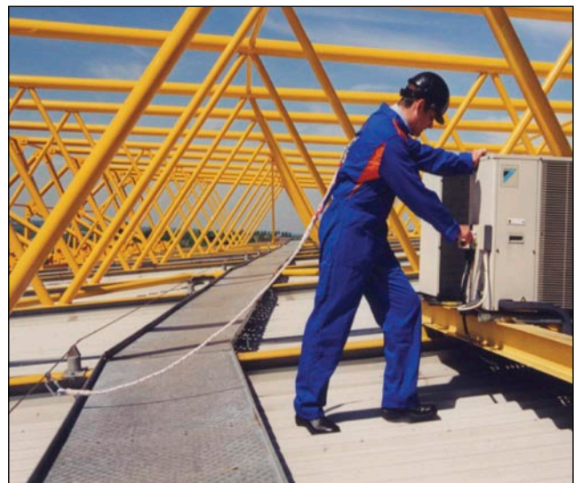
Figure 17 Work restraint harness used during short-term inspection on a flat roof (Image courtesy of Safesite Limited)
