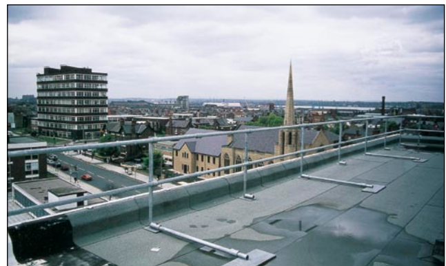
Figure 45 Permanent guard rail retrofitted during refurbishment work. Similar protection can be included in initial designs (Image courtesy of Safesite Limited)
