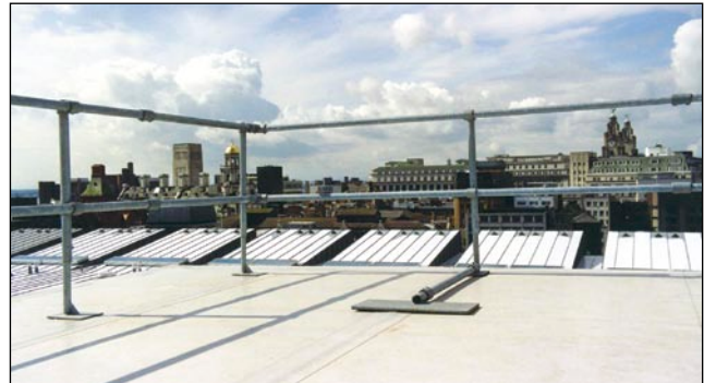
Figure 18 Temporary flat-roof edge protection. Adjustable supports enable work to progress with protection in place (Image courtesy of Safesite Limited)
