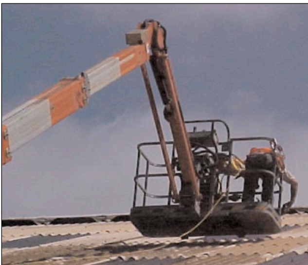
Figure 16 A mobile elevating work platform being used to replace a roof sheet
